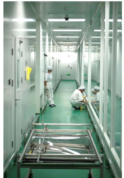
Careful consideration of process and space design to minimise costly high classification cleanroom areas.
