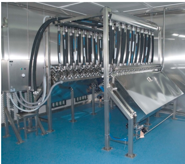
Powder handling lance racking system including CIP and SIP.
