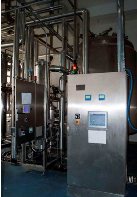
Extensive use of high purity nitrogen for O2 stripping and blanketing.
